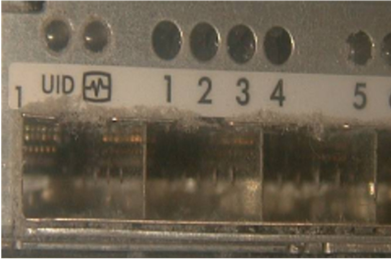
Figure 2.2 An example of unexpected dust accumulation around intakes. Particulate matter is shown in the small gap surrounding the connector sockets.
