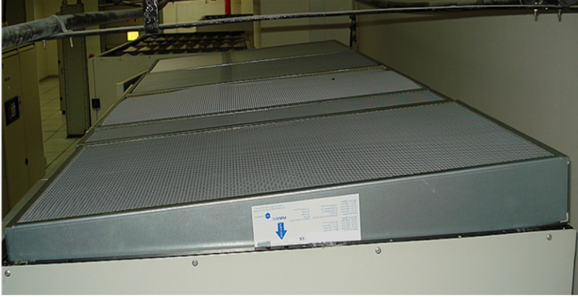
Figure 6.5 Combination particulate and chemical filter in CRAC unit with filter raised to show details.
