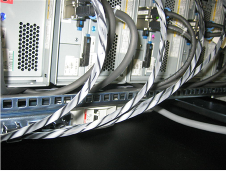
Figure 2.4 Sodium chloride dust on 220 Vac cables. The white deposits follow the high-electric-field pattern.
